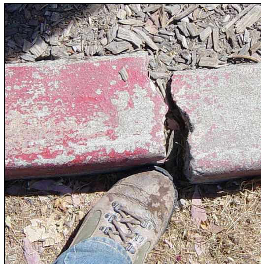
Fig. 3. ±15 years of curb displacement due to seismic-fault creep, Hayward Fault, Fremont, CA (photo courtesy of Wikipedia, in the public domain)
