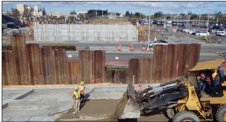
Fig. 4. Placing sand layer atop concrete load distribution slab constructed across Hayward Fault and beneath south abutment.
