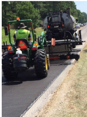
HaTelit® G50 being installed using PG 70-22 bitumen tack coat applied at a rate of approximately 0.12 gal sy. HaTelit® G50's unique material feature allows for direct installation on a milled surface.
