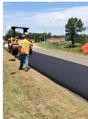
Final asphalt installation and compaction operation of the new 1.5" wearing course installed without any delays or issues by Barnhill Contracting.
