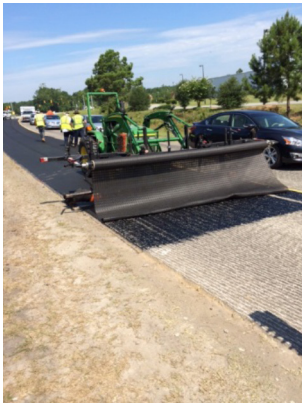
HaTelit® G50 installed on North Carolina State Route 130. HaTelit® G50 is being installed on a milled surface that had significant longitudinal, transverse and reflective cracking on the existing surface.
